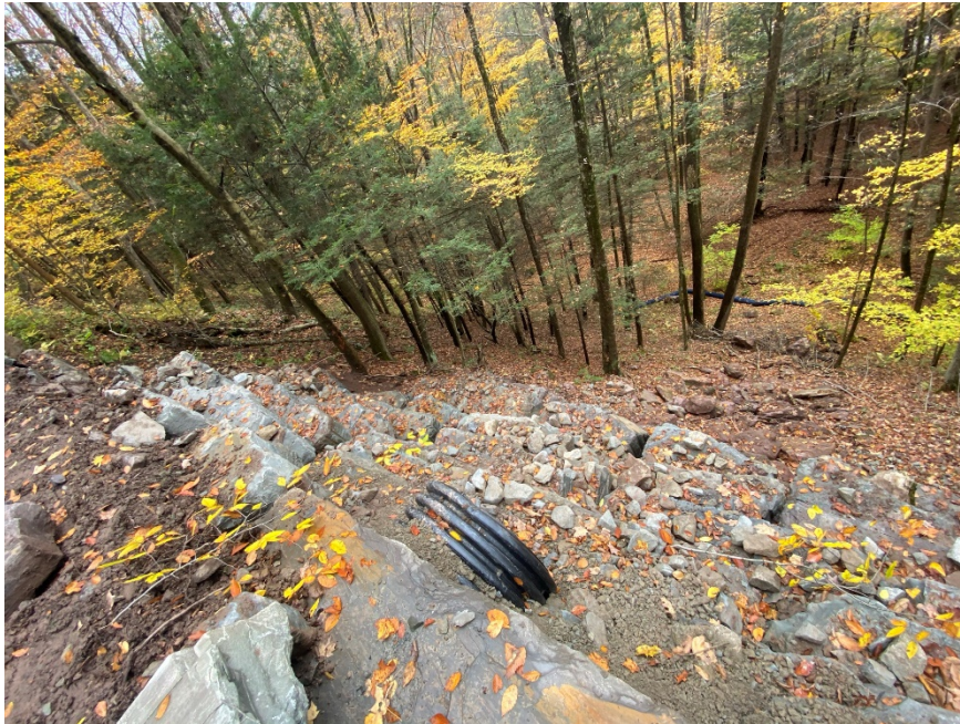
Image 3: View of rockery wall and drainage pipe from top of road, directly above rockery wall at Site 1 at Worlds End State Park
